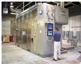
600kW 1st Gen Fuel Cell System
