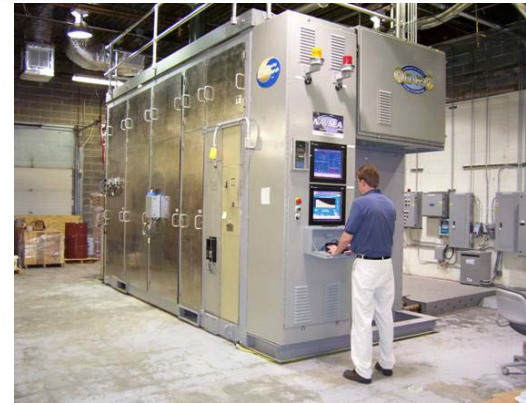
600 kW Reformer System Using High Sulfur Logistics Fuel
