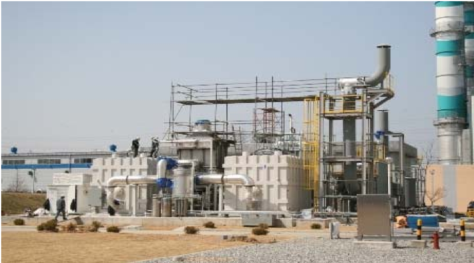
DFC 3000 (2.4 MW) - Gold Star Electric Power Station - Korea
