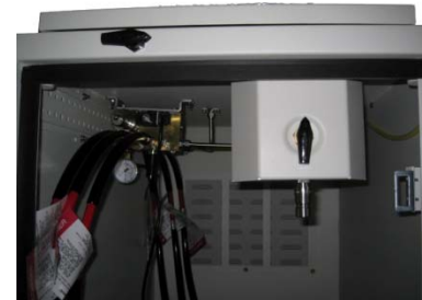
In-cabinet ground sites
