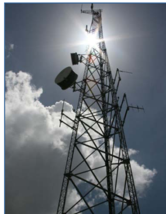
Hydrogen fuel cells providing critical backup power
