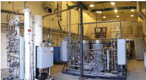
FIGURE 1. High pressure autothermal cyclic reforming (ACR) and PSA units. Installed at University of California, Irvine (UCI).
