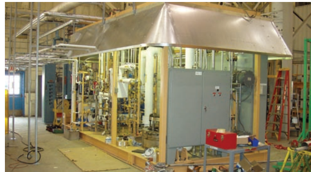
FIGURE 6. Small Hydrogen System Component Test Apparatus Installed at Praxair
