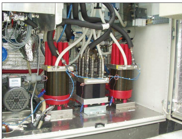
FIGURE 1. Proton's Cell Stacks on Site (the advanced 20/20 cell stack is in the middle)
