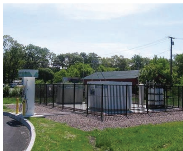
FIGURE 3. The Completed Station and Associated Equipment
