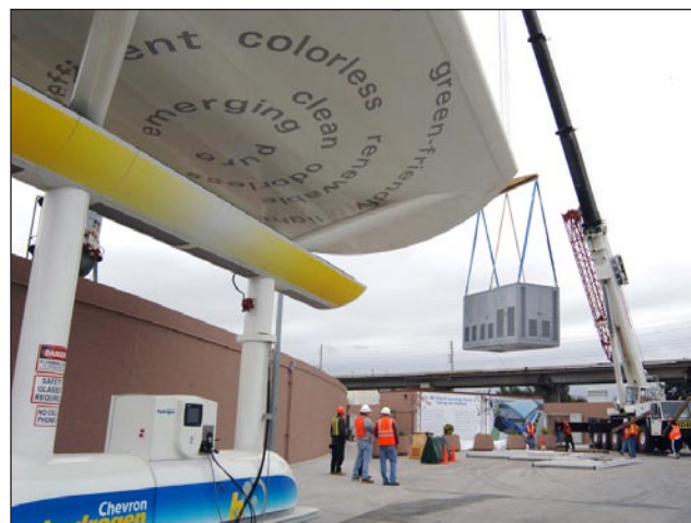
FIGURE 4. Infrastructure, Oakland Station
