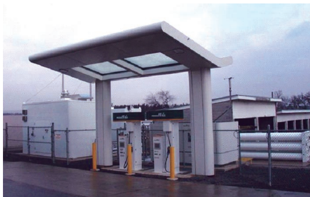
FIGURE 2. Equipment Installed at the Penn State H 2 Refueling Station
