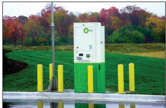
FIGURE 2. Hydrogen Dispenser, 5,000 psig
