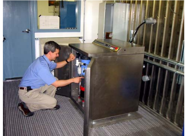
Figure 2. Hydrogen Electrolysis Test Facility - 5 kW PEM Electrolyzer
