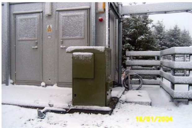
Figure 1. GC5T Installed at Host's Cell Tower
