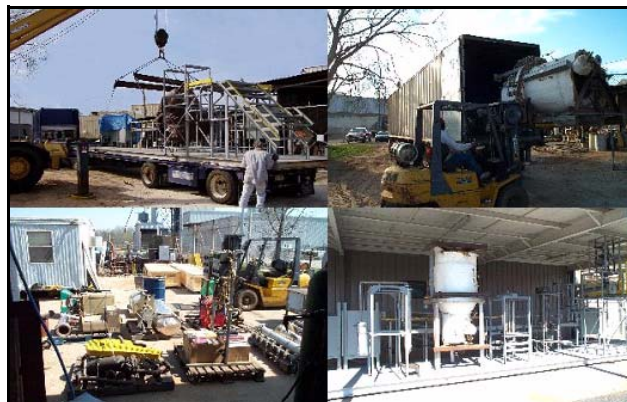
Figure 1. Pictures of the Pilot Plant Unit Being Moved and Reinstalled at Athens, Georgia
