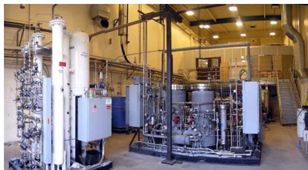
Figure 2. High Pressure Autothermal Cyclic Reforming (ACR) and PSA Units Installed at University of California, Irvine (UCI)
