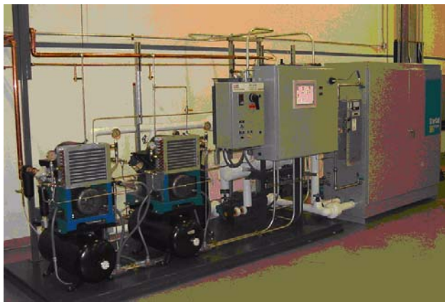
Figure 3. Installed StarCell System, July 2005
