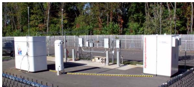
Figure 2. First Stage of Filling Station Undergoing Evaluation at Proton Energy Last Winter
