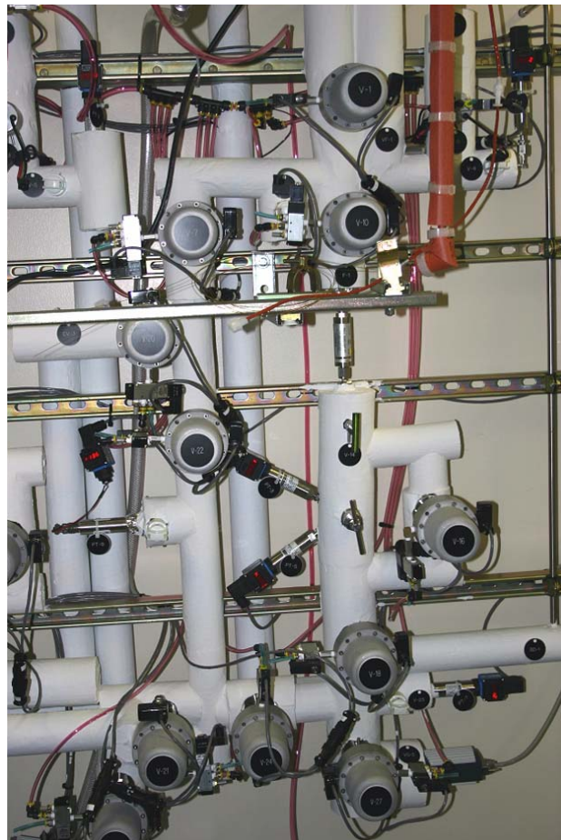
Figure 4. High Purity Gas Manifold with Capillary Fused Silica Gas Sampling Sub-Manifold
