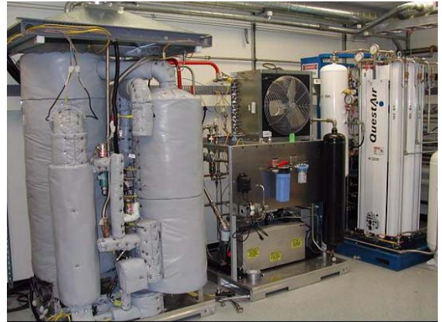
Figure 3. FP1A (left) and the Balance of Plant and PSA Subsystems in a System Level Evaluation
