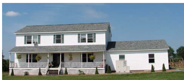
Figure 1. Residential Fuel Cell Installation in Upstate New York
