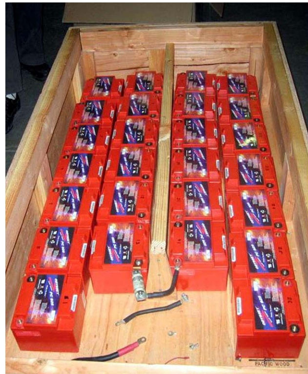
Figure 5. Battery Pack System used in the Hybrid Power Supply
