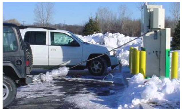
Figure 2. Dispenser Hose Breakaway Release Site Acceptance Test
