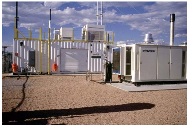
Figure 2. View of the Hydrogen Generator (Left) and Fuel Cell (Right)
