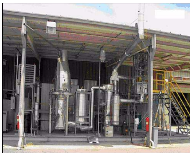
Figure 2. Photo of Pilot Scale Hydrogen Production Plant from Biomass
