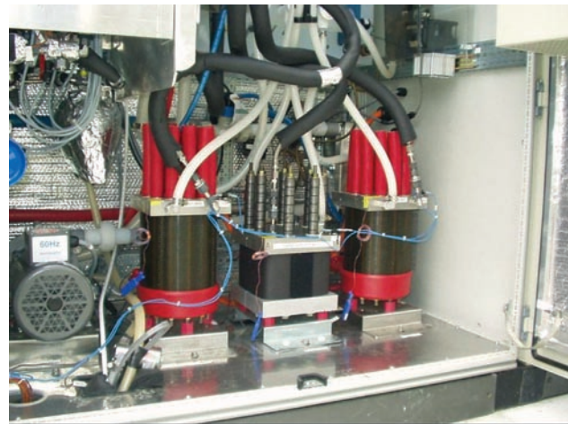
FIGURE 1. Proton Energy’s Cell Stacks On Site (the Advanced 20/20 Cell Stack is in the Middle)
