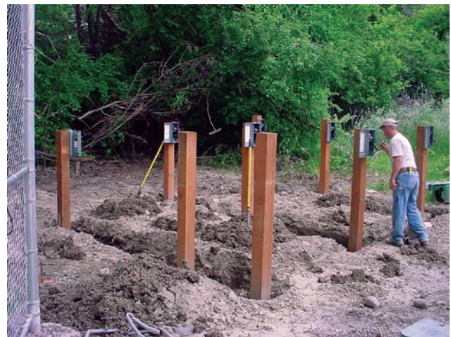
FIGURE 1. Fuel Cell Installation Site
