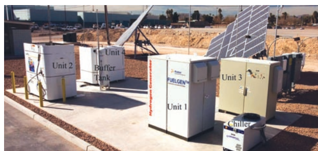
FIGURE 2. Equipment at the station includes: Unit 1 – the low pressure electrolyzer, Unit 2 – compressor/dispenser/storage, Unit 3 – high pressure electrolyzer, Unit 4 – compressor, chiller for Unit 4, buffer tank, with single-axis photovoltaic trackers in the background.
