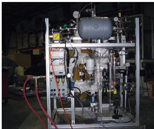
FIGURE 3. Mixer Showing H 2 and Water Control Systems
