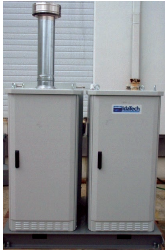
FIGURE 1. 5 kW net Indirect Methanol Fuel Cell Power Plant
