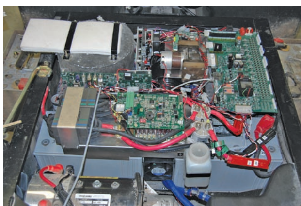
FIGURE 2. Upgraded IdaTech Liquid-Fueled Fuel Cell System Installed in TV-1
