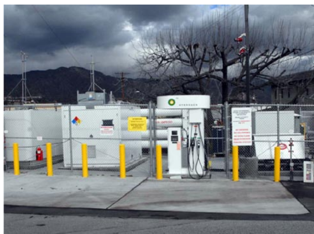
FIGURE 4. Burbank Hydrogen 35 MPa and 70 MPa Fueling Station
