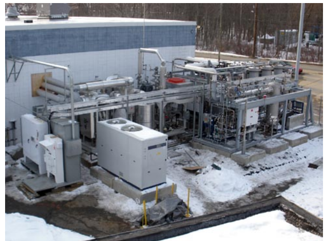
FIGURE 3. Hydrogen Energy Station Anode Exhaust and Hydrogen Purification Systems
