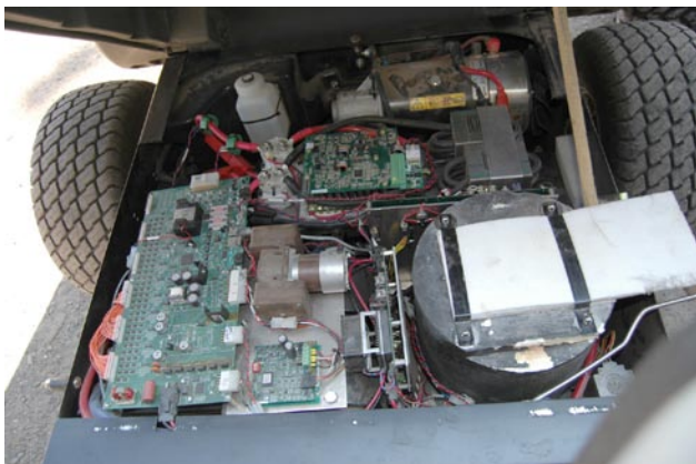
FIGURE 3. IdaTech Liquid Fueled Fuel Cell System Installed in TV-2
