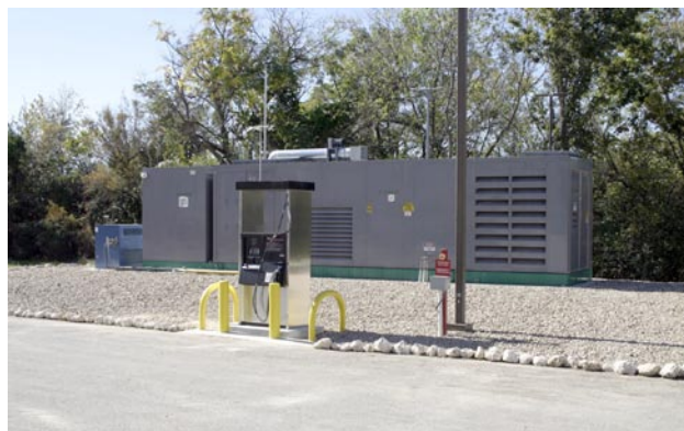
FIGURE 2. Hydrogen Fuel Station, Austin, Texas
