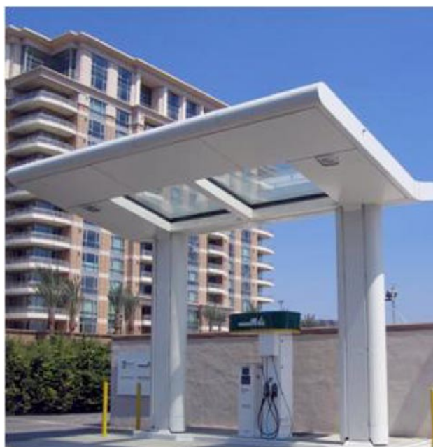
FIGURE 1. UCI 350/700 Bar Hydrogen Fueling Station
