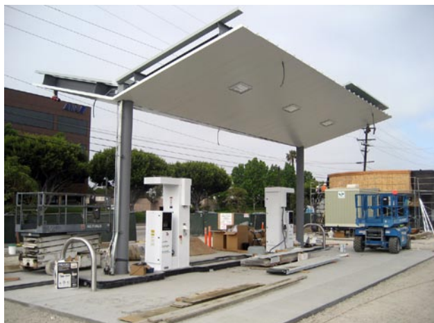
FIGURE 2. Torrance, CA Hydrogen Pipeline Fueling Station
