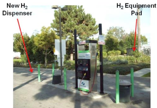
FIGURE 4. Fountain Valley Renewable Hydrogen Station
