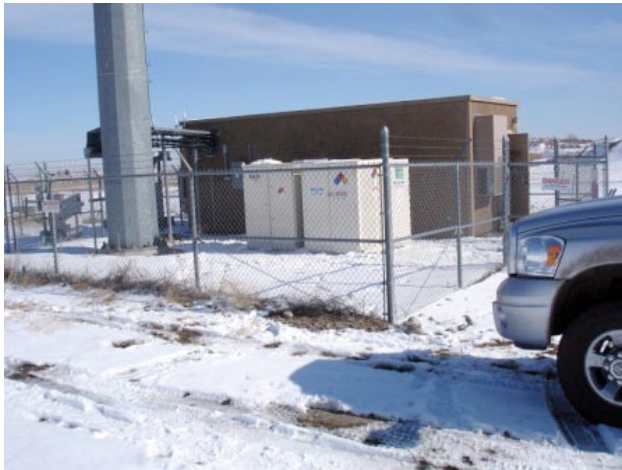
FIGURE 1. Completed AT&T Site (Arvada, CO)
