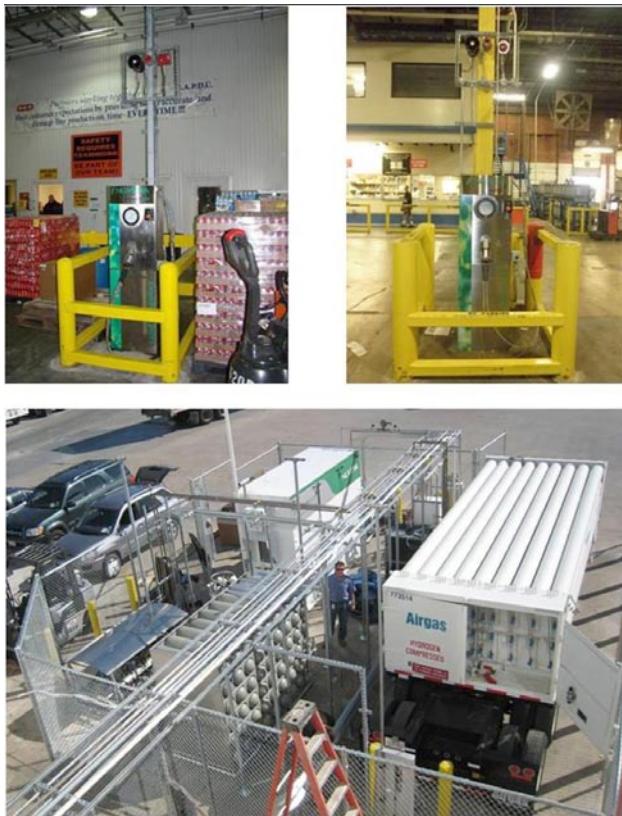
FIGURE 3. PowerTap™ Dispensers (top) and Generation, Compression, and Storage Equipment (bottom) for the H-E-B Fuel Cell Forklift Fleet
