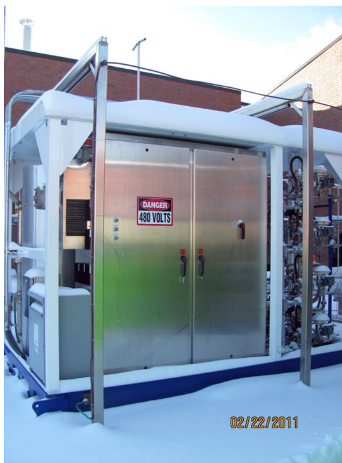
FIGURE 1. Desulfurizer Subsystem Being Tested in the Outdoor Test Facility (-23°C)
