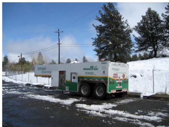
FIGURE 3. Air Products HF-150 Hydrogen Fueler – Placerville, CA
