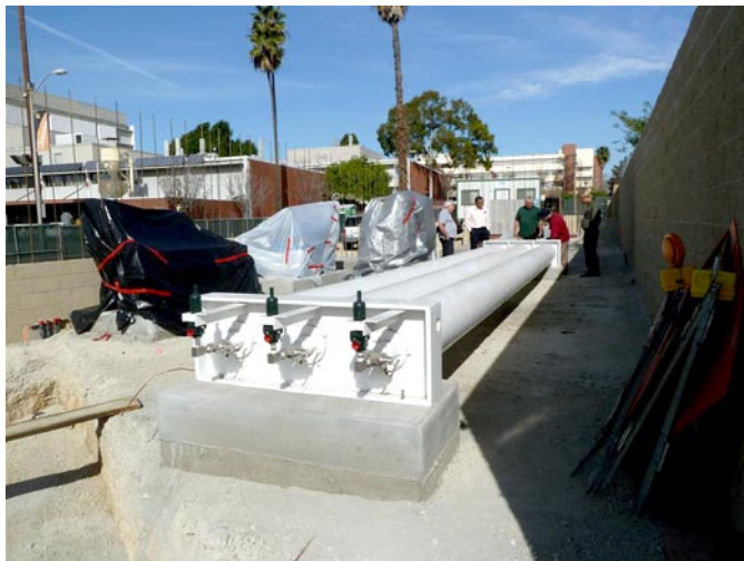
FIGURE 1. CSULA Hydrogen Fueling Facility, Compressors and Storage, January 2011
