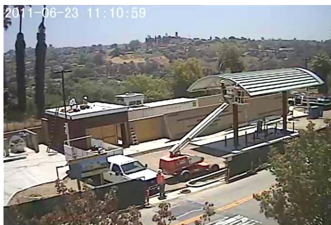
FIGURE 3. CSULA Hydrogen Fueling Facility, Current Status, June 2011
