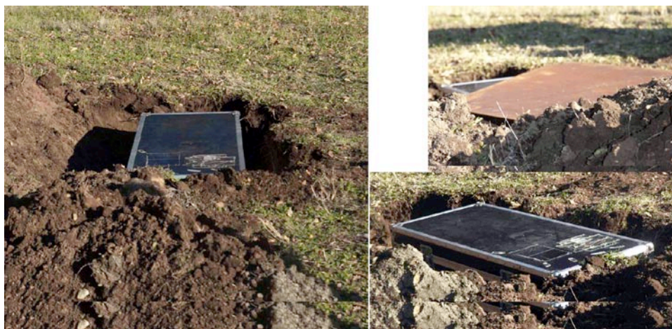
FIGURE 2. Photographs show ‘coffin’ emplacement and steel deck plate covering operations at SCC’s leased permeation test site. The coffin provides a clean environment for transportation (over dirt roads) and plumbing and data collection from a CPV under long duration testing with dangerous high-pressure fluids.
