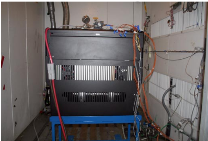
FIGURE 3. Final System Shown in Plug Power Environmental Testing Chamber
