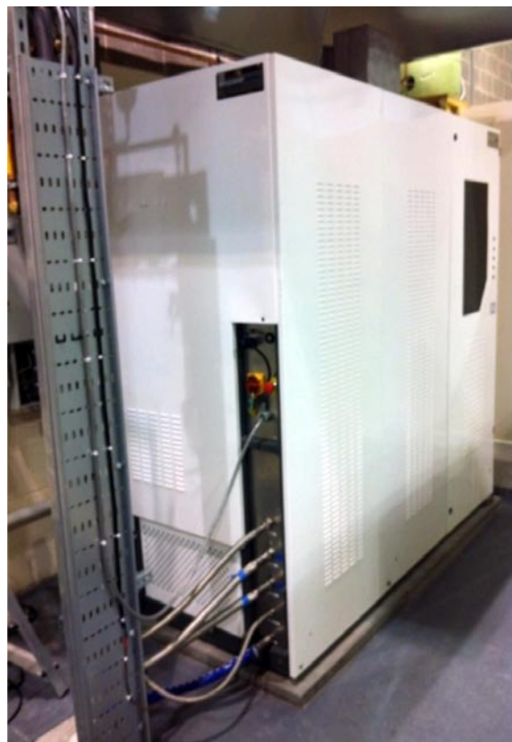
FIGURE 2. Packaged Demonstration Unit Installed
