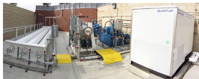
FIGURE 2. CSULA Hydrogen Fueling Facility, from left to right: storage tanks, PDC 350-bar bar compressor, two Hydro Pac 700-bar compressors, and Quantum chiller
