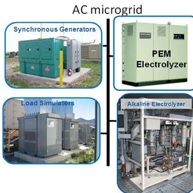
FIGURE 1. Frequency regulation experimental system where electrolyzers are powered by diesel generators on an AC microgrid
