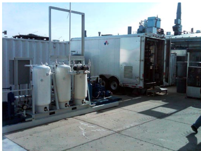
FIGURE 1. Gas clean-up skid and mobile hydrogen unit
