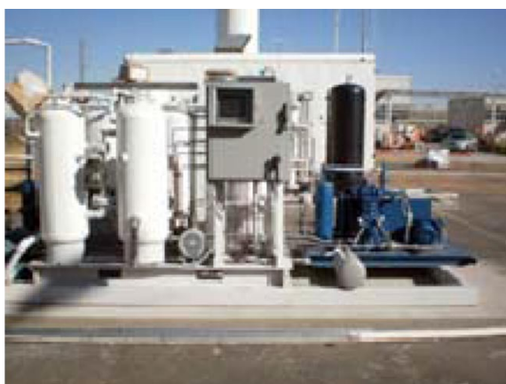
Landfill Gas Clean-Up Equipment November 26, 2012
