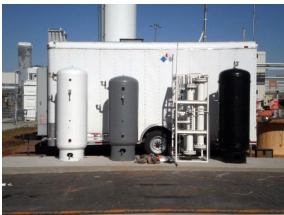
Hydrogen Generation Equipment November 12, 2012
