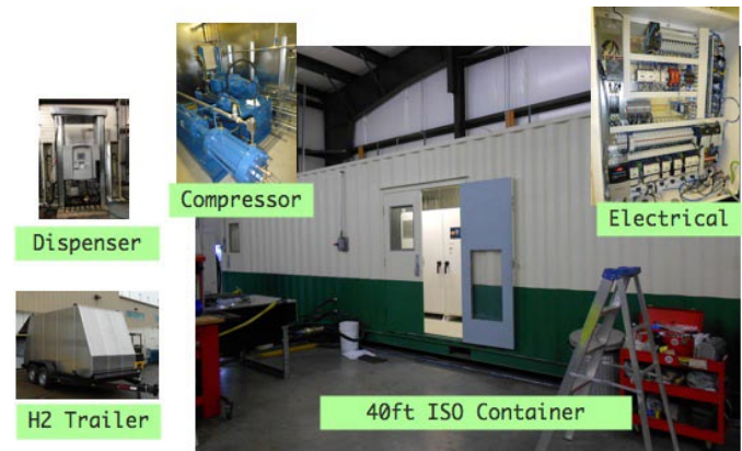
FIGURE 4. Hydrogen System Equipment
