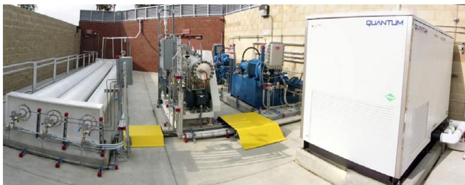
FIGURE 1. CSULA Hydrogen Fueling Facility, from left to right: storage tanks, PDC 350-bar compressor, two Hydro Pac 700-bar compressors, and Quantum chiller.
