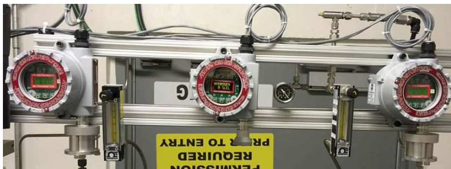
FIGURE 2. Leak detection system with fixed-area detector and two vacuum pump active sampling detectors
